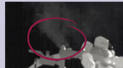
Captured SF 6 leak
